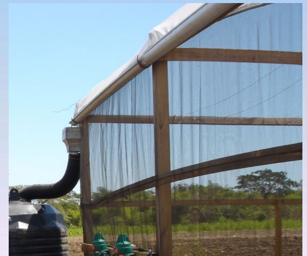
Guttering system to facilitate rainwater harvesting
